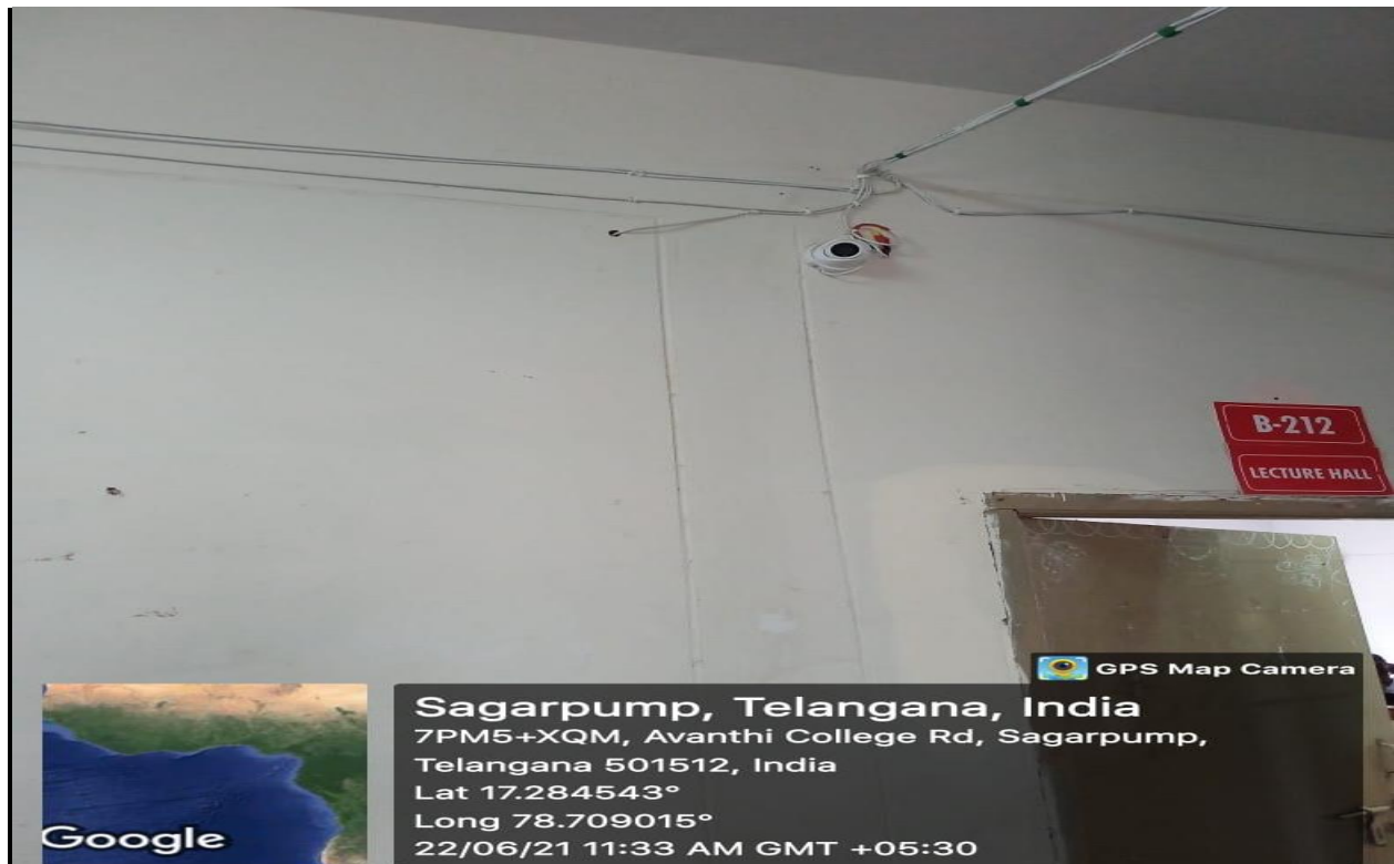
|CC-Camera at Lecture hall , First floor
